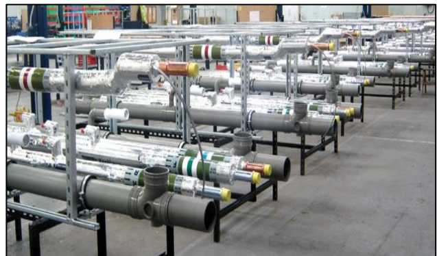
Figure 3 A modularization shop where the components are built in a control environment. Image courtesy of http://www.mepsolutions.com
