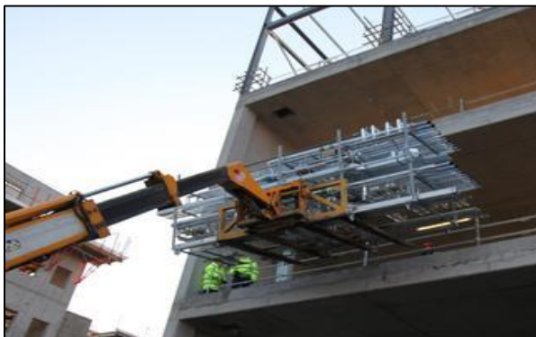
Figure 4 The installation process of the MEP system modular. Image courtesy of http://www.globaloff-site.com
